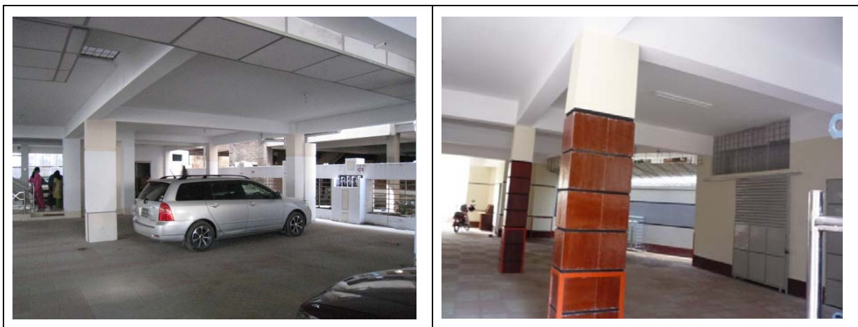
Figure 2-8 Ground floor being Used as Car Park: One of the Typical Buildings in Dhaka
