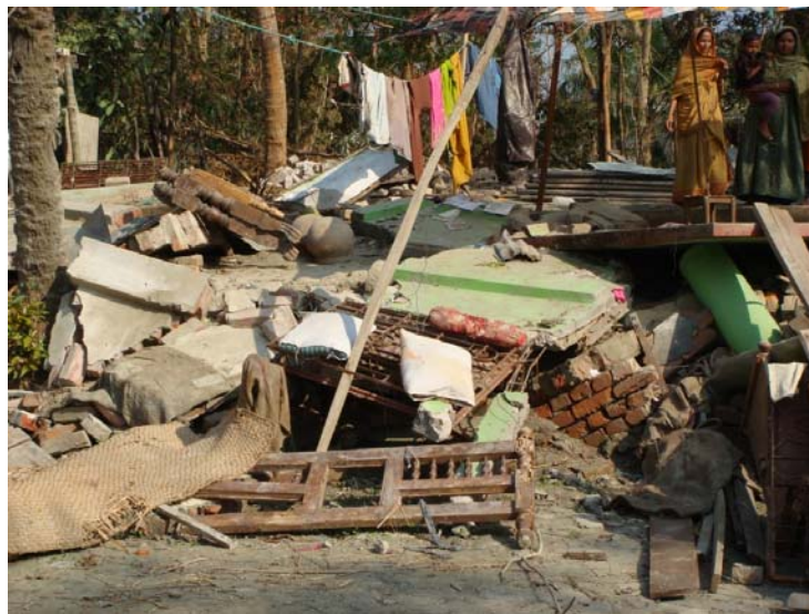
Photo 12.1: A masonry structure completely collapsed due to storm-surge during Cyclone Sidr in 2007
