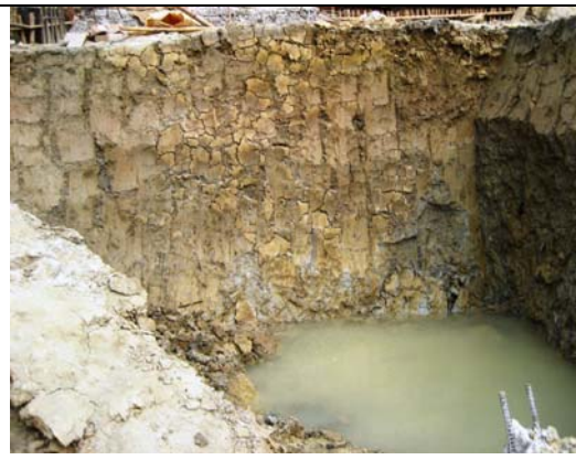
Photo-2.24. Section at Konapara (DND) bus stand. Section shows soft clay of Lower Kalsi Bed.
