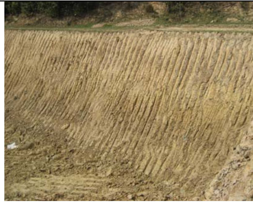
Photo-2.22. Section at Shaheengarh, Pubail, Lower Kalsi Bed. Thick deposit of yellowish-brown swelling clay
