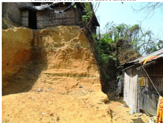
Vulnerable houses at Mohajer para
