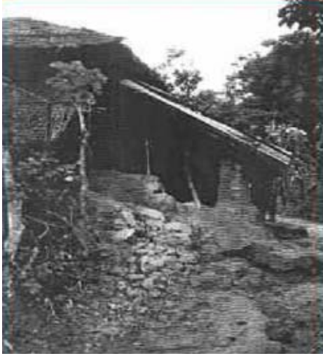
Damage to house in 1997 Earthquake in Moshekhali
