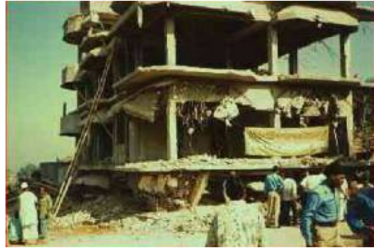
Damage to an under construction building in Chittagong City in 1997
