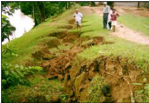
Landslide, Kalabunia, Rangamati after 2003 EQ
