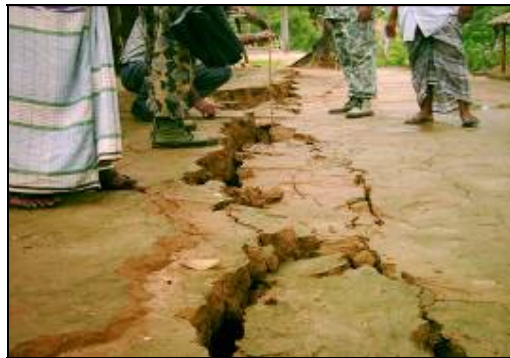
Big Crack on the earthen Road at BDR CAMP, after 2003 EQ
