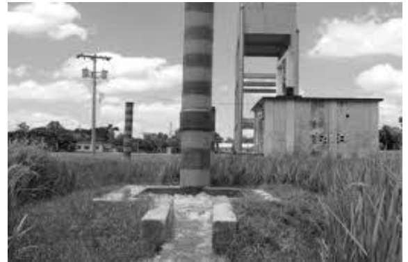
Figure1.4:Deep tubewell under borendro irrigation project
