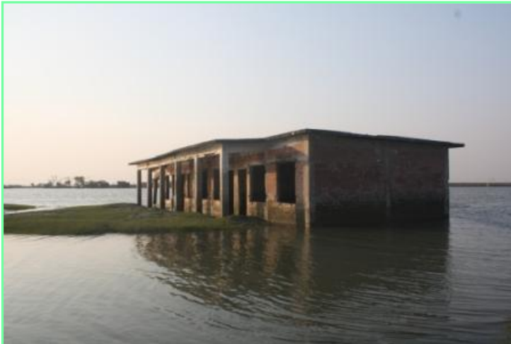
Unruly River is slowly engulfing the Bainpara Primary School piece by piece. For safety the school is shifted to another temporary location
